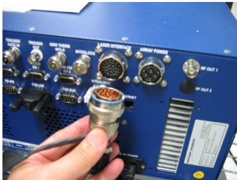
Figure 4-10 Laser Signal Cable
